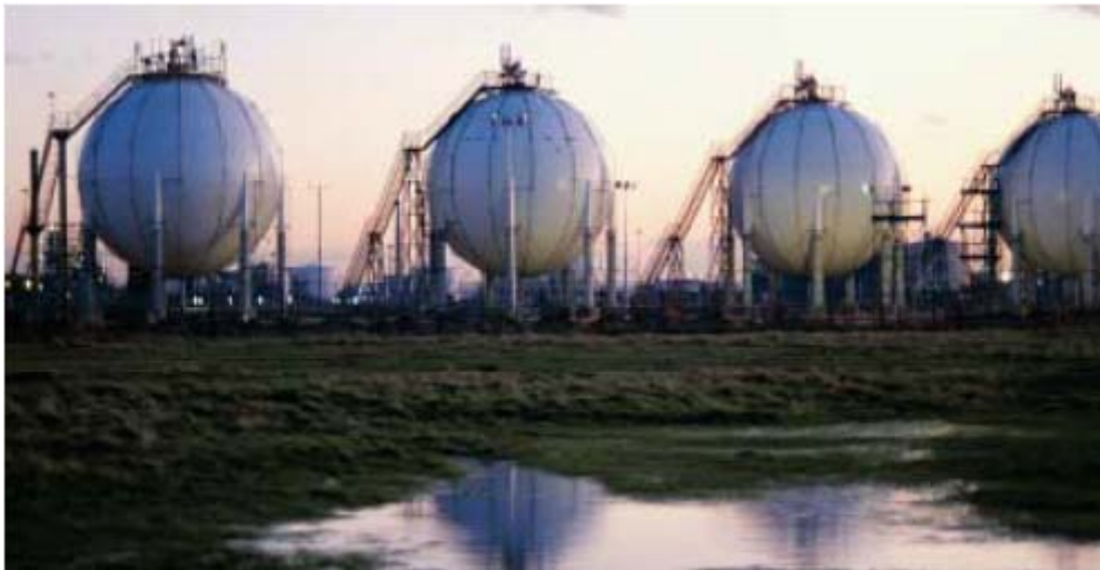
Figure 14: Above-Ground Natural Gas Storage Facilities
